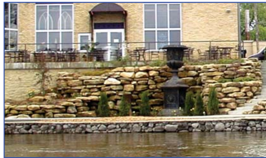
River Walks are an important community assets in many of our Rock River Stormwater Group communities, including Fort Atkinson pictured here. Floodwaters have devastated a number of these riverwalks in the past. By working together these communities are striving to have water stay where it lands, infiltrating into the ground and not contributing to the stormwater woes.
